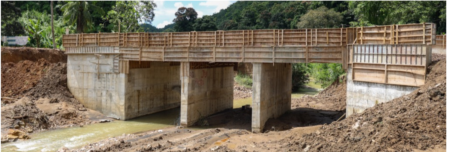
TROY BRIDGE POST HURRICANE MELISSA
